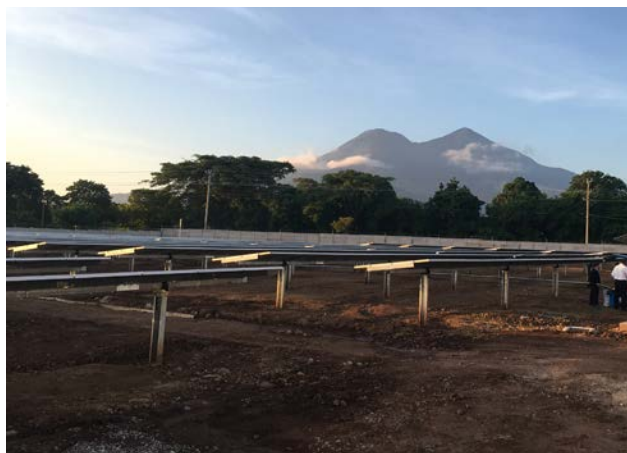
Single-axis solar PV tracking system in Central America (Photo credit: Laird Reed)
