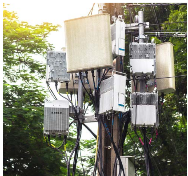
Wireless broadband infrastructure (Photo credit: Shutterstock)
